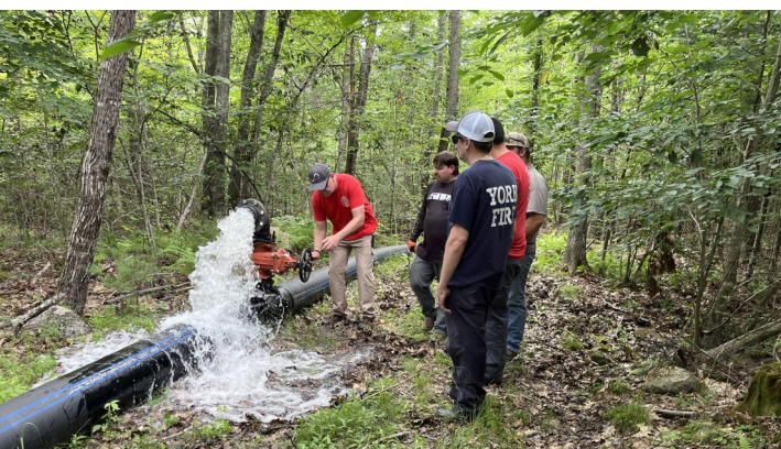
Fire Department testing out the dry hydrant on the syphon line.
